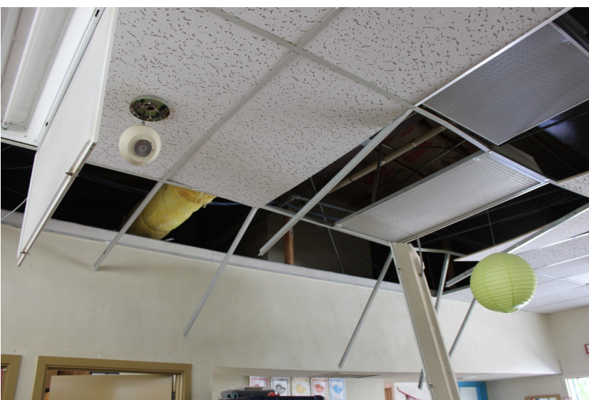
This photo was taken in Ridgecrest CA after a series of earthquakes in 2019. Although the building structure itself did not suffer damage, portions of the ceiling system failed, causing dangerous conditions for occupants and a considerable amount of debris throughout the room.
